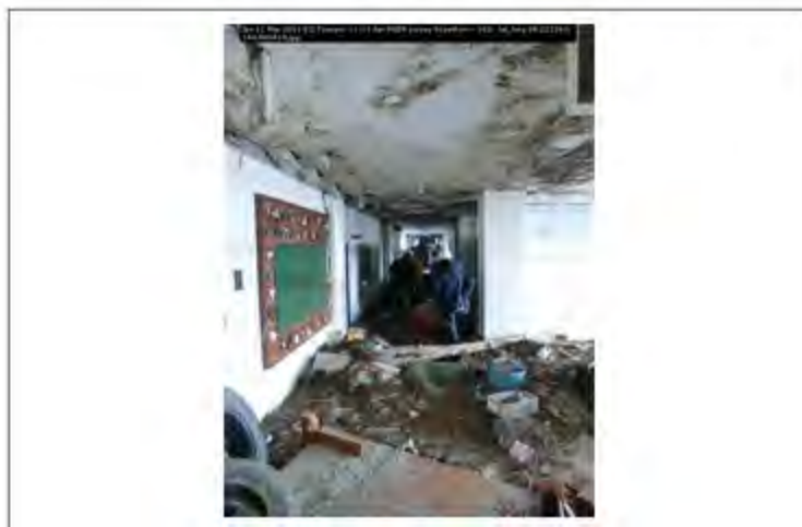
Jpn 11 Mar 2011 EQ Tsunami 11-13 Apr PEER survey Scawthorn - 162; lat_long 38.222268; 140.980418
