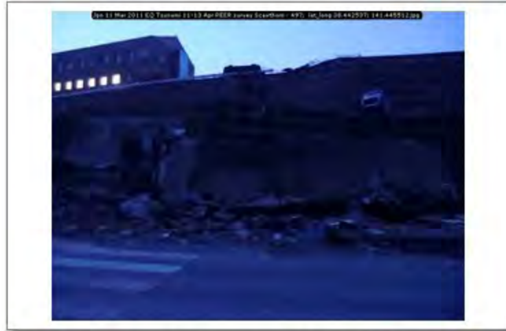
Jpn 11 Mar 2011 EQ Tsunami 11-13 Apr PEER survey Scawthorn - 497; lat_long 38.442537; 141.445512
