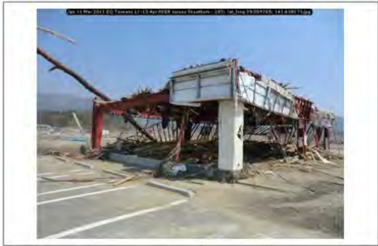
Jpn 11 Mar 2011 EQ Tsunami 11-13 Apr PEER survey Scawthorn - 287; lat_long 39.009765; 141.638173
