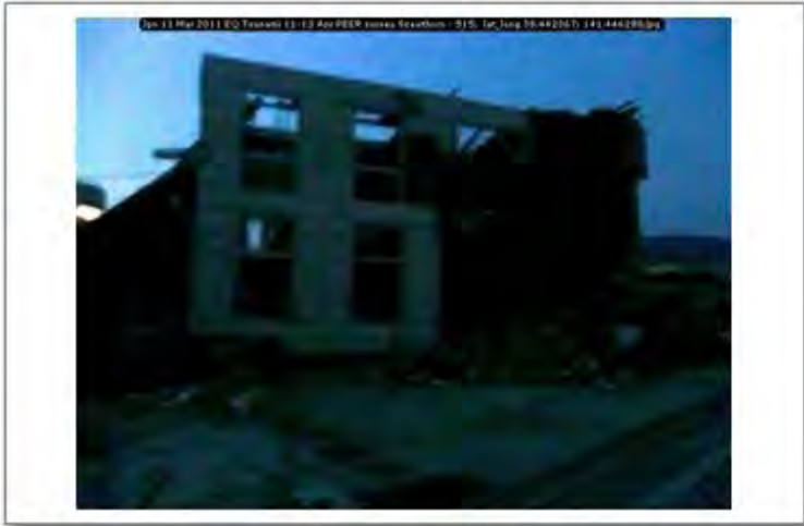
Jpn 11 Mar 2011 EQ Tsunami 11-13 Apr PEER survey Scawthorn - 515; lat_long 38.442367; 141.446288
