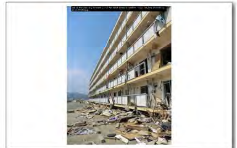
Jpn 11 Mar 2011 EQ Tsunami 11-13 Apr PEER survey Scawthorn - 322; lat_long 39.009772; 141.645193
