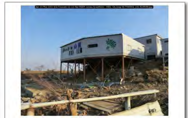
Jpn 11 Mar 2011 EQ Tsunami 11-13 Apr PEER survey Scawthorn - 480; lat_long 38.794583; 141.528588
