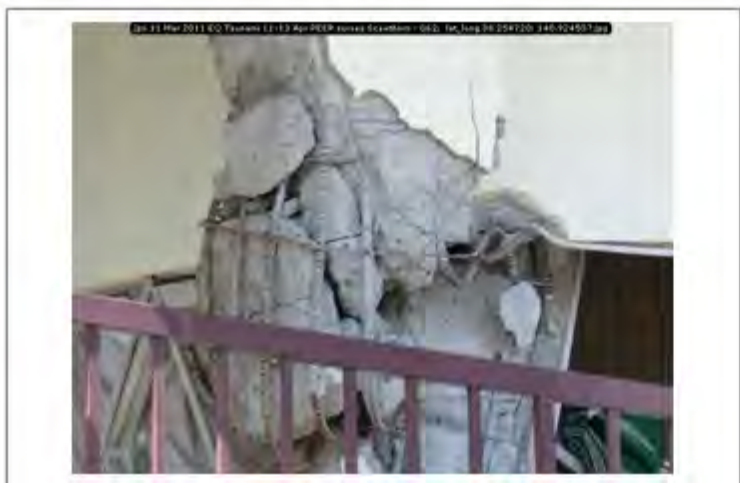
Jpn 11 Mar 2011 EQ Tsunami 11-13 Apr PEER survey Scawthorn - 062; lat_long 38.254720; 140.924507
