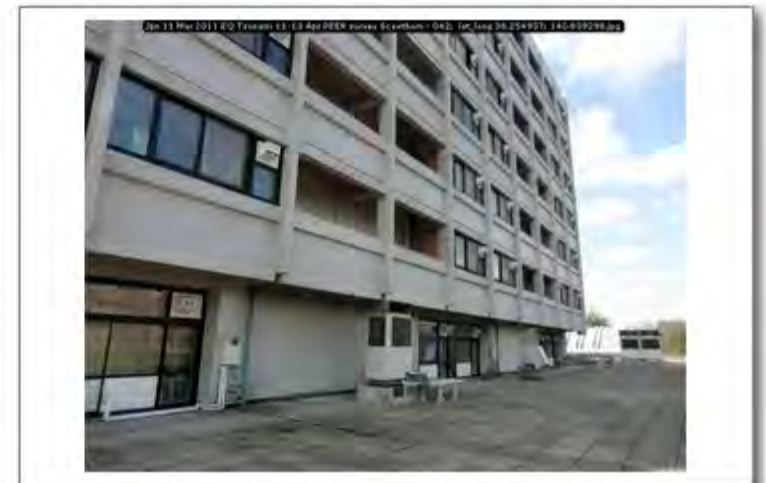
Jpn 11 Mar 2011 EQ Tsunami 11-13 Apr PEER survey Scawthorn - 042; lat_long 38.254937; 140.839298
