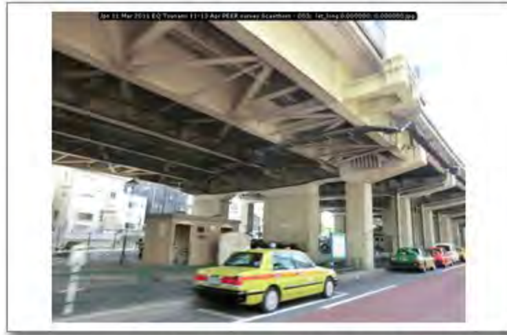
Jpn 11 Mar 2011 EQ Tsunami 11-13 Apr PEER survey Scawthorn - 003; lat_long 0.000000; 0.000000
