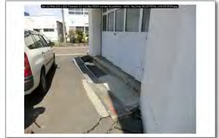
Jpn 11 Mar 2011 EQ Tsunami 11-13 Apr PEER survey Scawthorn - 083; lat_long 38.257550; 140.937828
