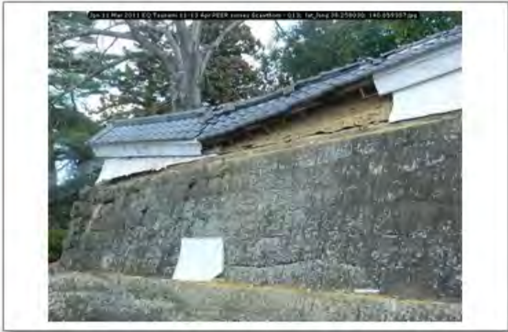
Jpn 11 Mar 2011 EQ Tsunami 11-13 Apr PEER survey Scawthorn - 013; lat_long 38.258030; 140.859307
