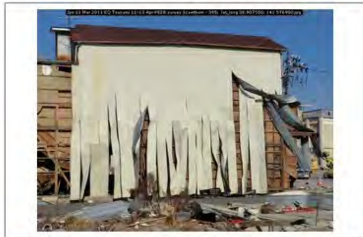
Jpn 11 Mar 2011 EQ Tsunami 11-13 Apr PEER survey Scawthorn - 395; lat_long 38.907550; 141.576900
