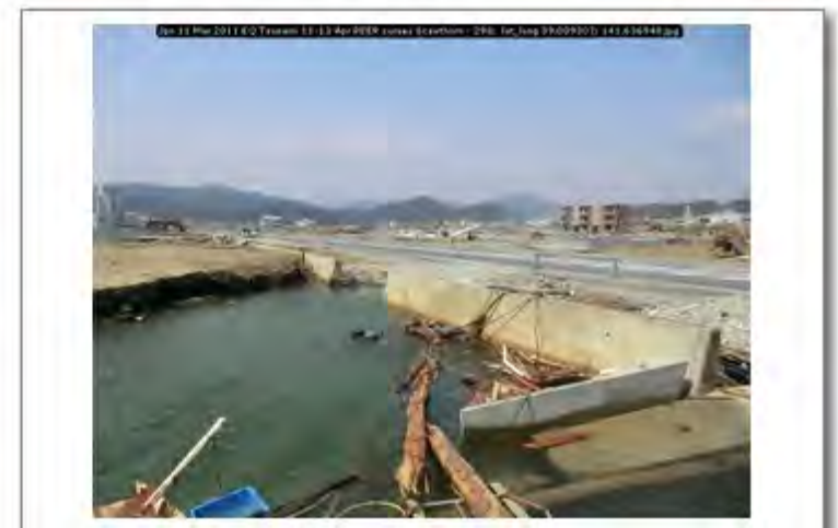
Jpn 11 Mar 2011 EQ Tsunami 11-13 Apr PEER survey Scawthorn - 298; lat_long 39.009307; 141.636948
