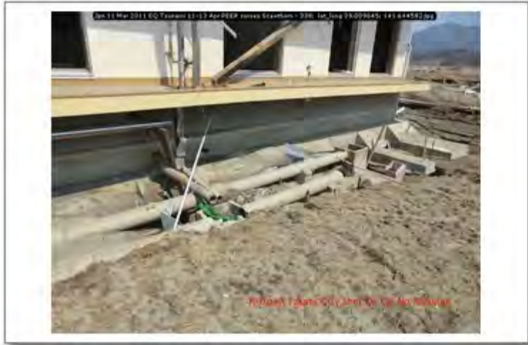
Jpn 11 Mar 2011 EQ Tsunami 11-13 Apr PEER survey Scawthorn - 338; lat_long 39.009645; 141.644582
