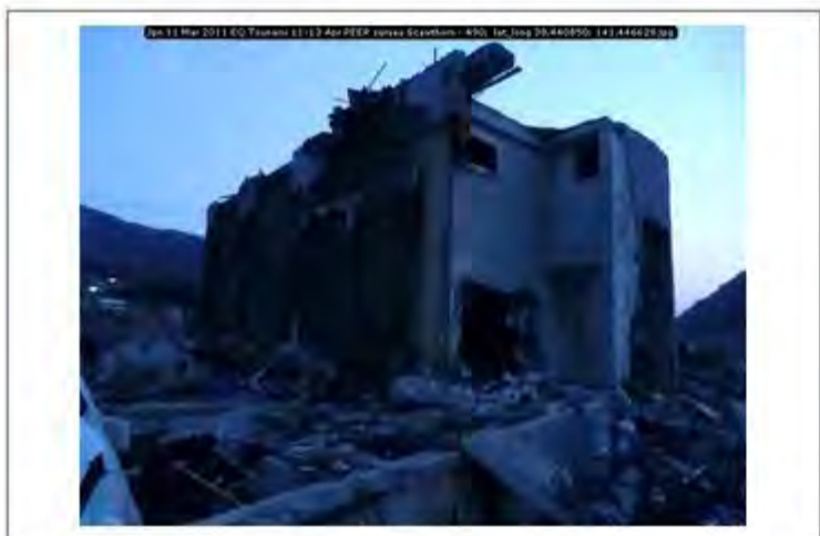
Jpn 11 Mar 2011 EQ Tsunami 11-13 Apr PEER survey Scawthorn - 490; lat_long 38.440850; 141.446628
