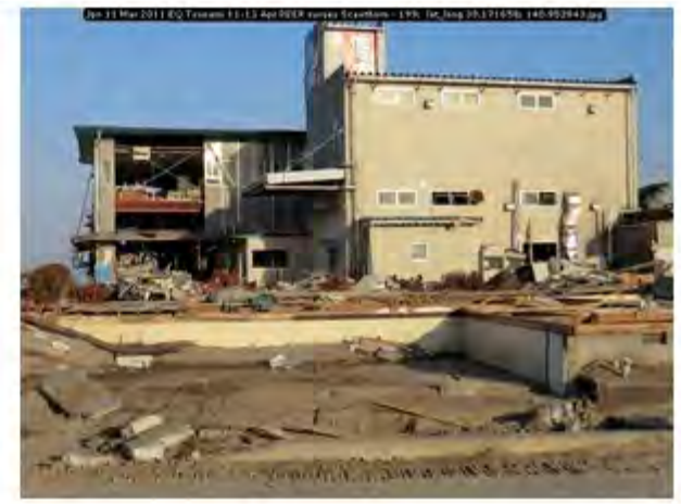
Jpn 11 Mar 2011 EQ Tsunami 11-13 Apr PEER survey Scawthorn - 199; lat_long 38.171658; 140.952843
