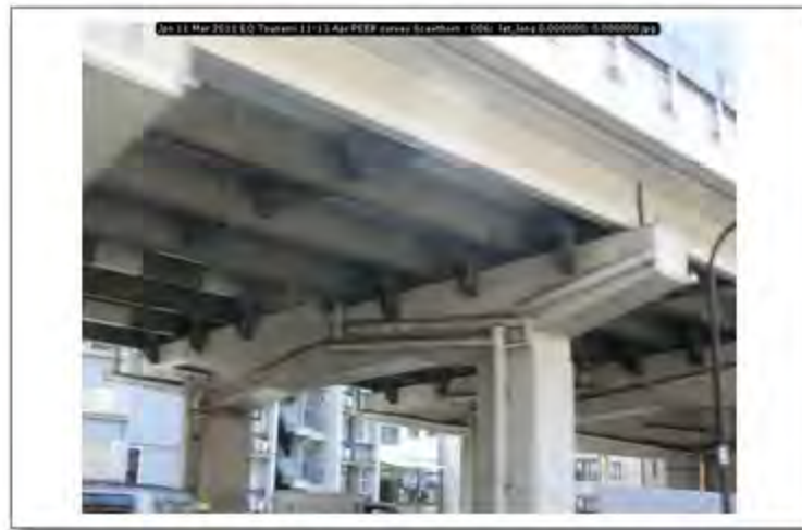
Jpn 11 Mar 2011 EQ Tsunami 11-13 Apr PEER survey Scawthorn - 006; lat_long 0.000000; 0.000000
