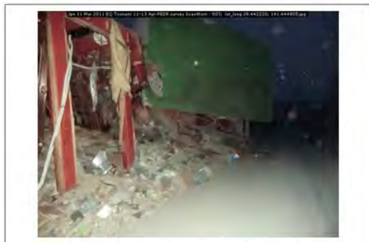
Jpn 11 Mar 2011 EQ Tsunami 11-13 Apr PEER survey Scawthorn - 507; lat_long 38.442220; 141.444805
