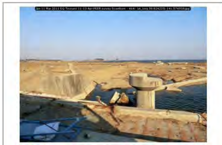
Jpn 11 Mar 2011 EQ Tsunami 11-13 Apr PEER survey Scawthorn - 464; lat_long 38.824225; 141.574938
