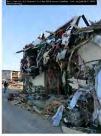
Jpn 11 Mar 2011 EQ Tsunami 11-13 Apr PEER survey Scawthorn - 194; lat_long 38.171955; 140.952902
