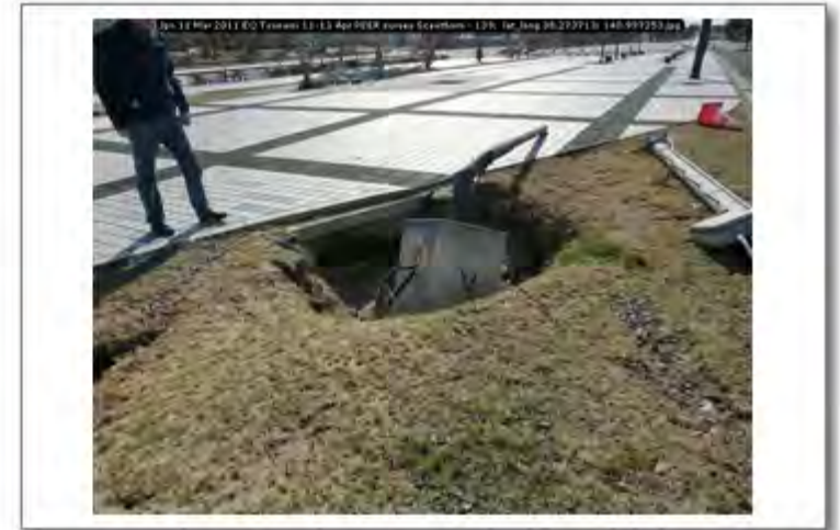
Jpn 11 Mar 2011 EQ Tsunami 11-13 Apr PEER survey Scawthorn - 139; lat_long 38.273713; 140.997253
