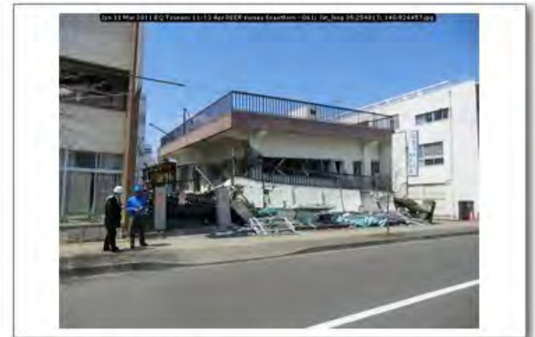
Jpn 11 Mar 2011 EQ Tsunami 11-13 Apr PEER survey Scawthorn - 061; lat_long 38.254817; 140.924457
