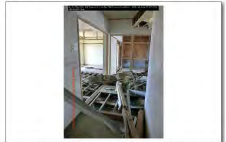
Jpn 11 Mar 2011 EQ Tsunami 11-13 Apr PEER survey Scawthorn - 325; lat_long 39.009872; 141.644717
