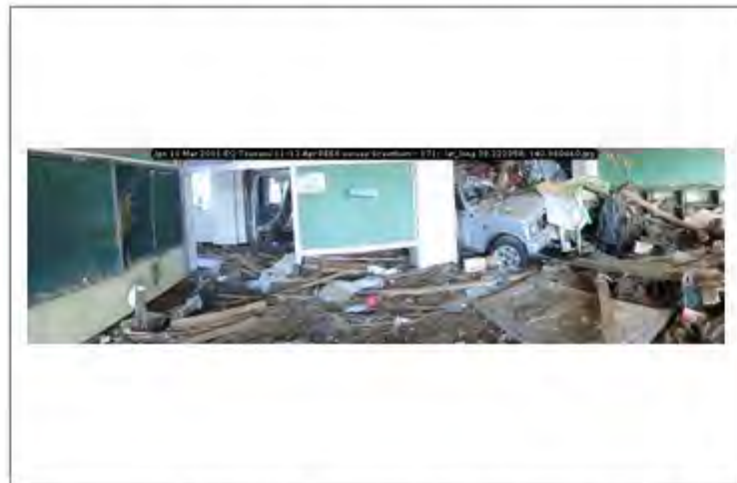
Jpn 11 Mar 2011 EQ Tsunami 11-13 Apr PEER survey Scawthorn - 171; lat_long 38.222358; 140.980660
