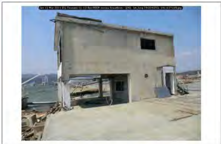
Jpn 11 Mar 2011 EQ Tsunami 11-13 Apr PEER survey Scawthorn - 290; lat_long 39.009253; 141.637165
