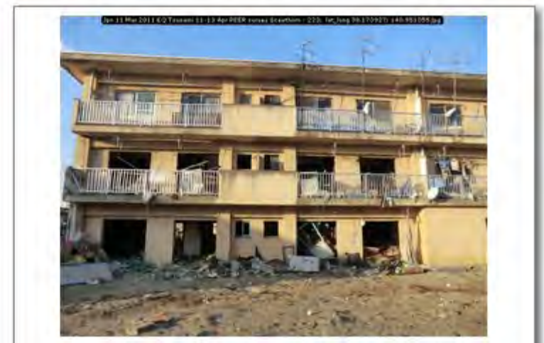
Jpn 11 Mar 2011 EQ Tsunami 11-13 Apr PEER survey Scawthorn - 223; lat_long 38.170927; 140.951055
