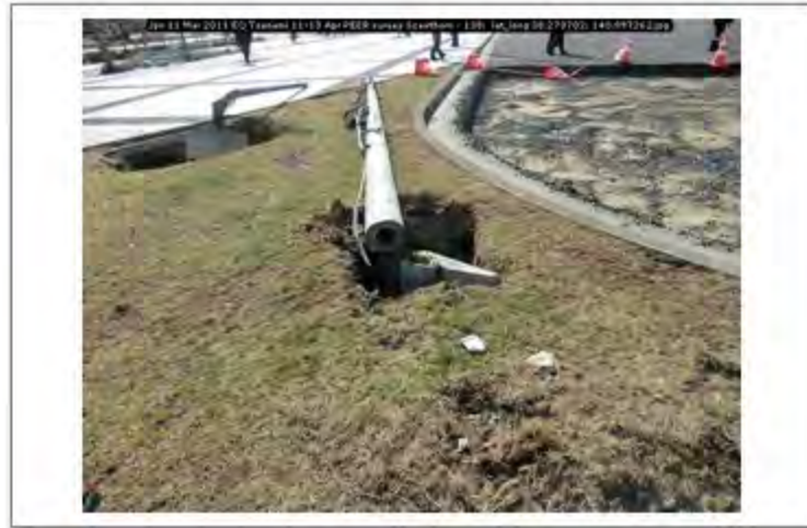
Jpn 11 Mar 2011 EQ Tsunami 11-13 Apr PEER survey Scawthorn - 138; lat_long 38.273702; 140.997262
