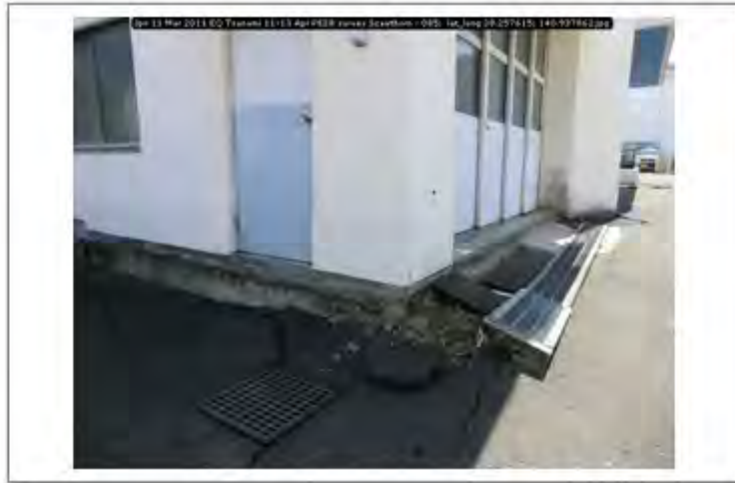
Jpn 11 Mar 2011 EQ Tsunami 11-13 Apr PEER survey Scawthorn - 085; lat_long 38.257615; 140.937862
