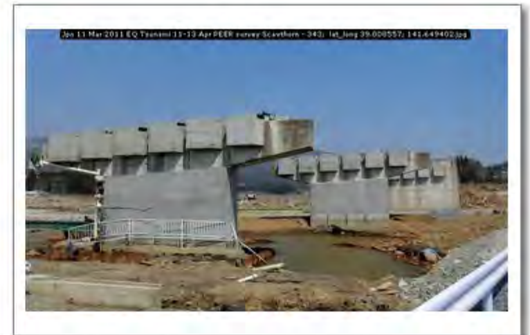
Jpn 11 Mar 2011 EQ Tsunami 11-13 Apr PEER survey Scawthorn - 343; lat_long 39.008557; 141.649402
