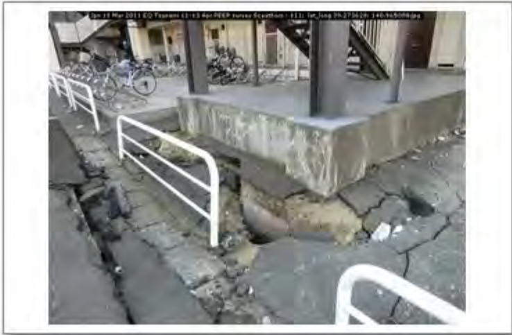
Jpn 11 Mar 2011 EQ Tsunami 11-13 Apr PEER survey Scawthorn - 111; lat_long 38.273628; 140.965088
