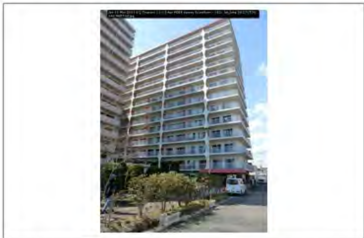
Jpn 11 Mar 2011 EQ Tsunami 11-13 Apr PEER survey Scawthorn - 102; lat_long 38.271530; 140.965732
