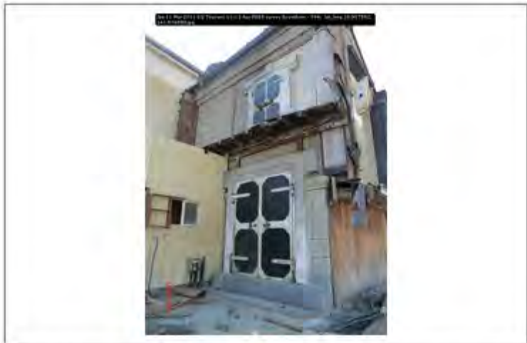
Jpn 11 Mar 2011 EQ Tsunami 11-13 Apr PEER survey Scawthorn - 394; lat_long 38.907552; 141.576893
