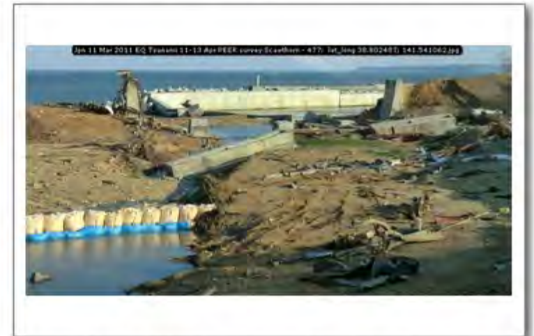
Jpn 11 Mar 2011 EQ Tsunami 11-13 Apr PEER survey Scawthorn - 477; lat_long 38.802487; 141.541062
