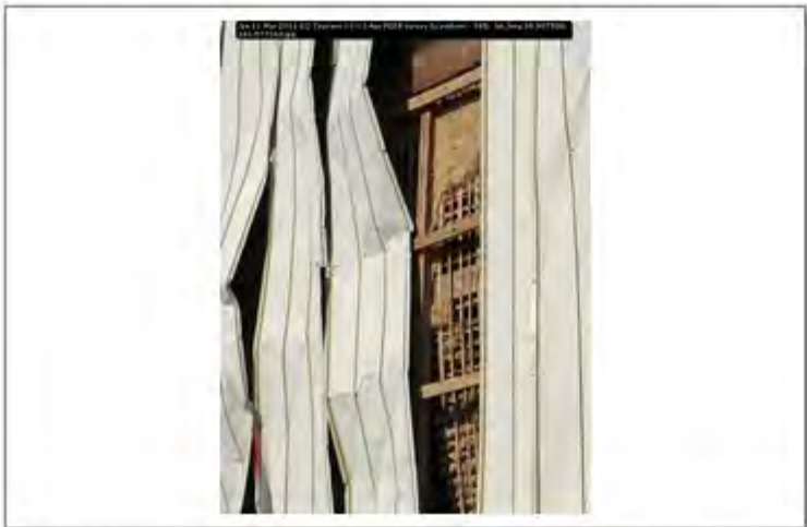
Jpn 11 Mar 2011 EQ Tsunami 11-13 Apr PEER survey Scawthorn - 385; lat_long 38.907500; 141.577248
