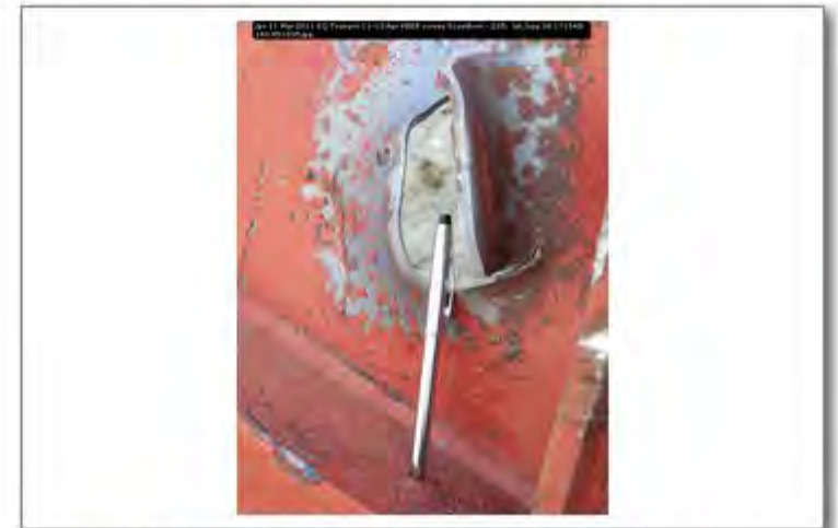
Jpn 11 Mar 2011 EQ Tsunami 11-13 Apr PEER survey Scawthorn - 235; lat_long 38.171548; 140.951035
