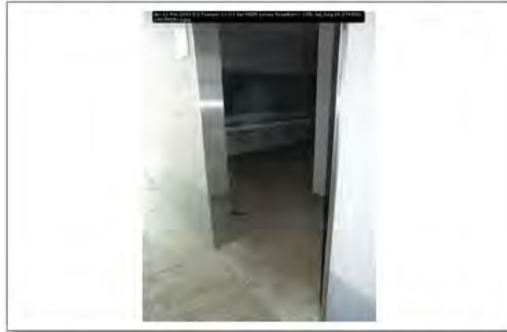
Jpn 11 Mar 2011 EQ Tsunami 11-13 Apr PEER survey Scawthorn - 135; lat_long 38.274300; 140.995812
