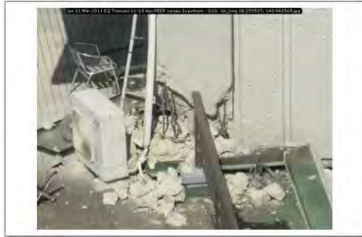
Jpn 11 Mar 2011 EQ Tsunami 11-13 Apr PEER survey Scawthorn - 020; lat_long 38.255537; 140.842565
