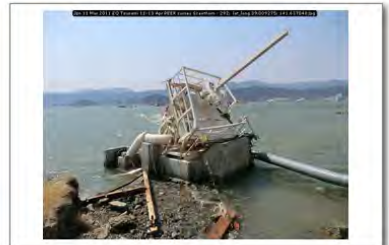
Jpn 11 Mar 2011 EQ Tsunami 11-13 Apr PEER survey Scawthorn - 292; lat_long 39.009275; 141.637048
