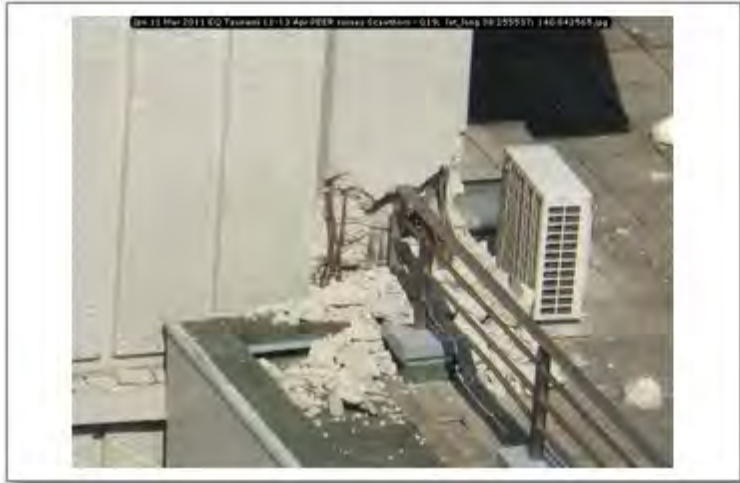
Jpn 11 Mar 2011 EQ Tsunami 11-13 Apr PEER survey Scawthorn - 019; lat_long 38.255537; 140.842565
