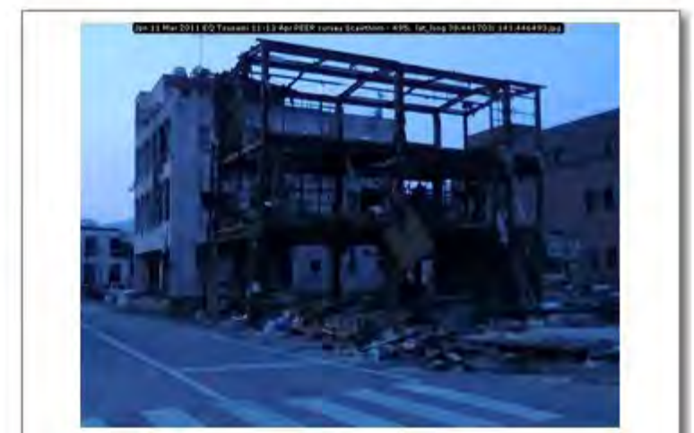
Jpn 11 Mar 2011 EQ Tsunami 11-13 Apr PEER survey Scawthorn - 495; lat_long 38.441703; 141.446493
