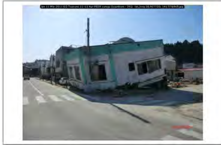
Jpn 11 Mar 2011 EQ Tsunami 11-13 Apr PEER survey Scawthorn - 392; lat_long 38.907720; 141.576865
