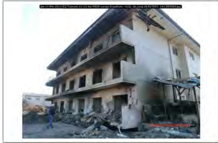
Jpn 11 Mar 2011 EQ Tsunami 11-13 Apr PEER survey Scawthorn - 422; lat_long 38.917557; 141.583580
