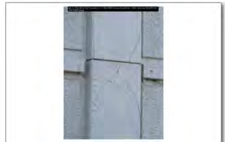
Jpn 11 Mar 2011 EQ Tsunami 11-13 Apr PEER survey Scawthorn - 048; lat_long 38.255143; 140.838313
