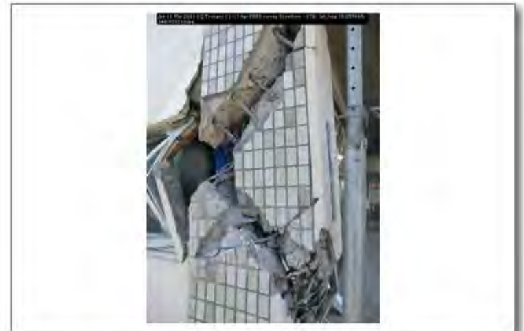
Jpn 11 Mar 2011 EQ Tsunami 11-13 Apr PEER survey Scawthorn - 070; lat_long 38.259845; 140.923210
