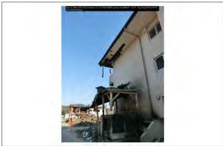
Jpn 11 Mar 2011 EQ Tsunami 11-13 Apr PEER survey Scawthorn - 419; lat_long 38.917647; 141.583232
