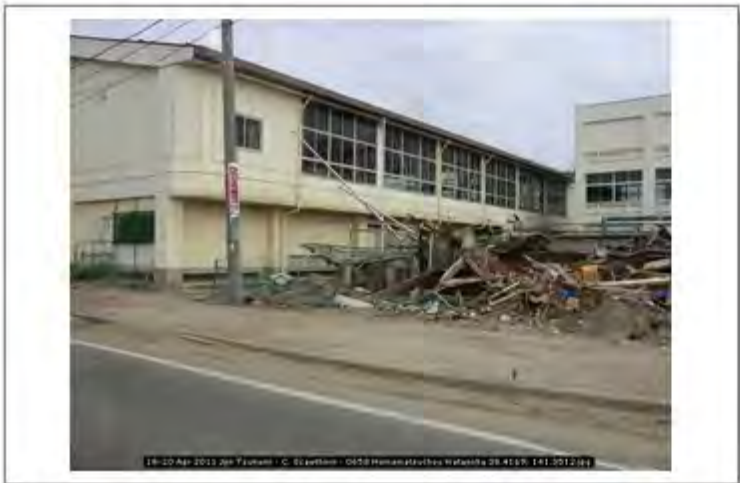
18-20 Apr 2011 Jpn Tsunami - C. Scawthorn - 0658 Hamamatsuchou Watanoha 38.4169; 141.3512
