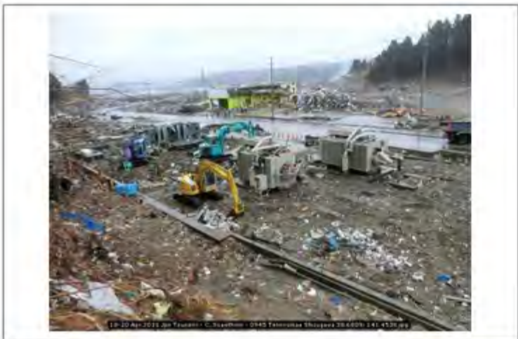
18-20 Apr 2011 Jpn Tsunami - C. Scawthorn - 0945 Tennoumae Shizugawa 38.6809; 141.4538
