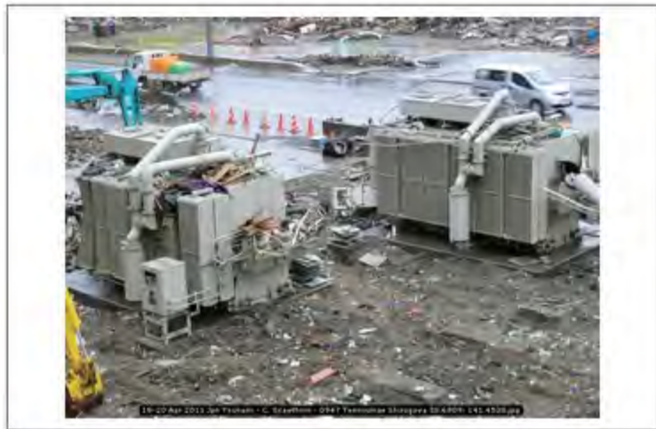
18-20 Apr 2011 Jpn Tsunami - C. Scawthorn - 0947 Tennoumae Shizugawa 38.6809; 141.4538
