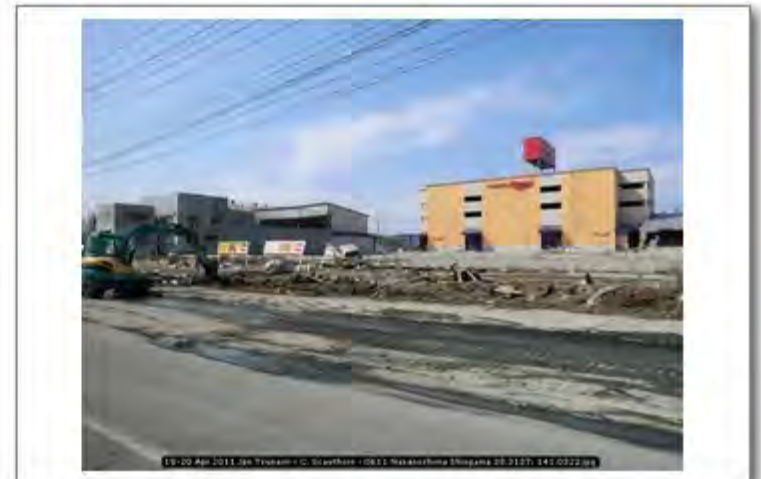
18-20 Apr 2011 Jpn Tsunami - C. Scawthorn - 0611 Nakanoshima Shiogama 38.3137; 141.0322
