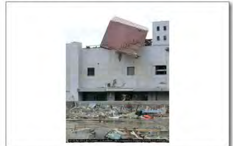
18-20 Apr 2011 Jpn Tsunami - C. Scawthorn - 0671 Koganechou Onagawa 38.4435; 141.4468
