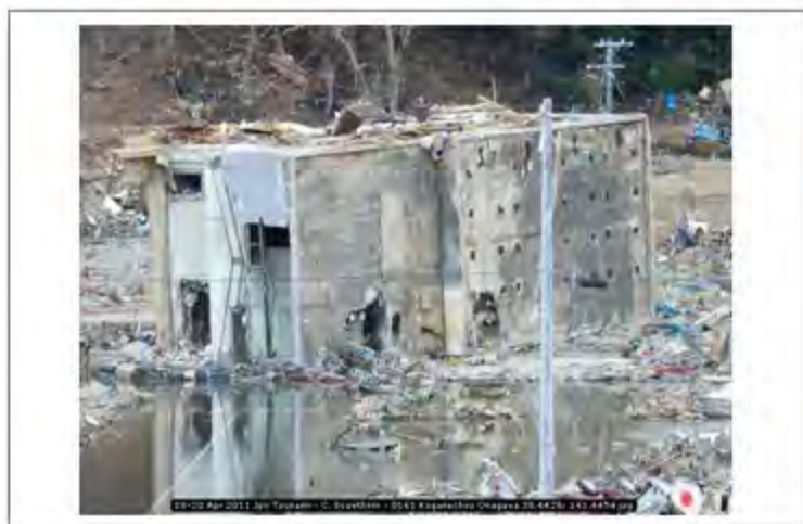
18-20 Apr 2011 Jpn Tsunami - C. Scawthorn - 0161 Koganechou Onagawa 38.4428; 141.4454
