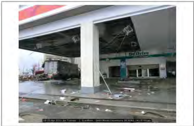
18-20 Apr 2011 Jpn Tsunami - C. Scawthorn - 0469 Minato Kesennuma 38.9040; 141.5799
