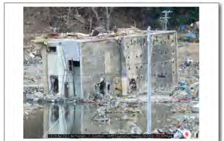
18-20 Apr 2011 Jpn Tsunami - C. Scawthorn - 0695 Koganechou Onagawa 38.4428; 141.4454
