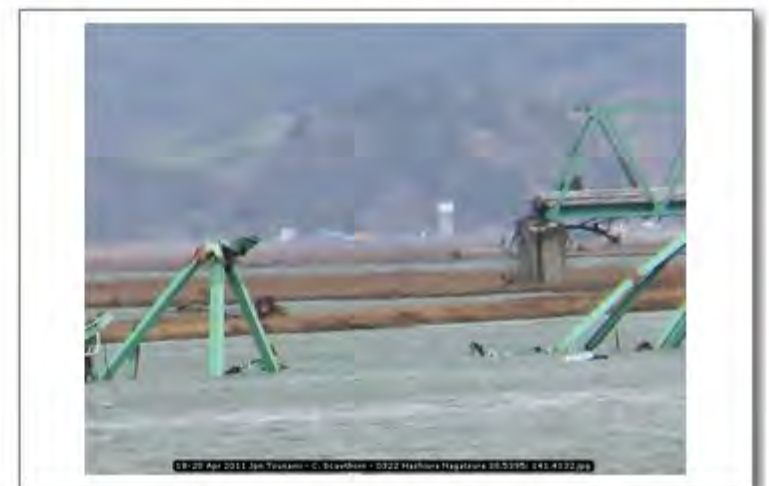
18-20 Apr 2011 Jpn Tsunami - C. Scawthorn - 0322 Hashiura Nagatsura 38.5395; 141.4132
