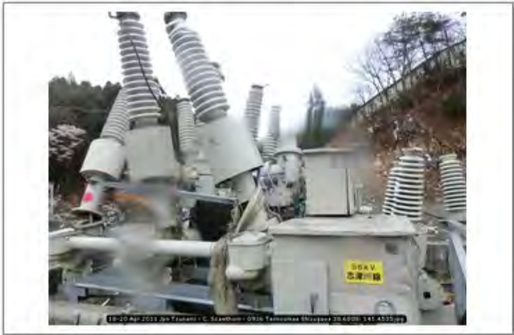
18-20 Apr 2011 Jpn Tsunami - C. Scawthorn - 0936 Tennoumae Shizugawa 38.6808; 141.4535
