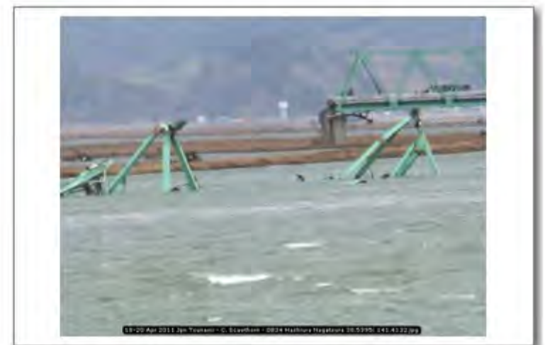
18-20 Apr 2011 Jpn Tsunami - C. Scawthorn - 0834 Hashiura Nagatsura 38.5395; 141.4132
