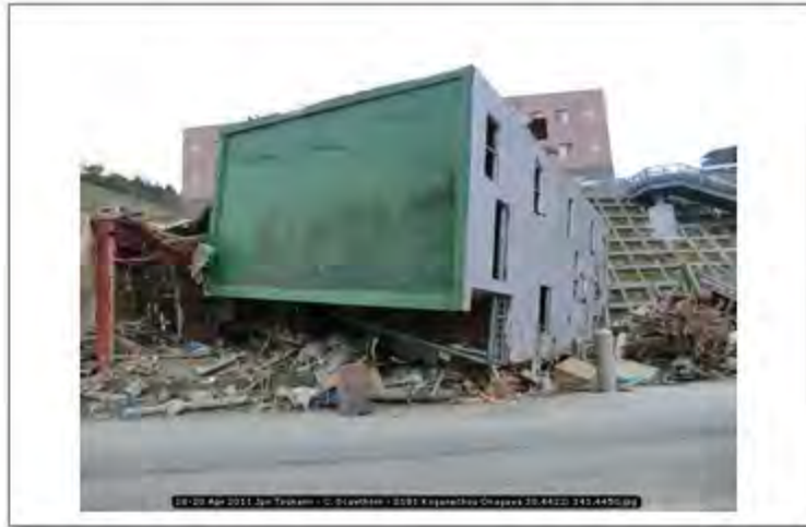
18-20 Apr 2011 Jpn Tsunami - C. Scawthorn - 0181 Koganechou Onagawa 38.4422; 141.4450
