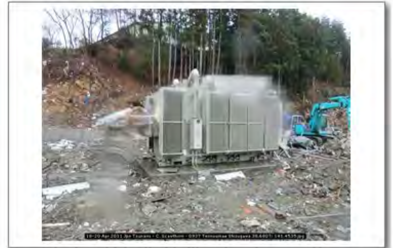
18-20 Apr 2011 Jpn Tsunami - C. Scawthorn - 0937 Tennoumae Shizugawa 38.6807; 141.4535
