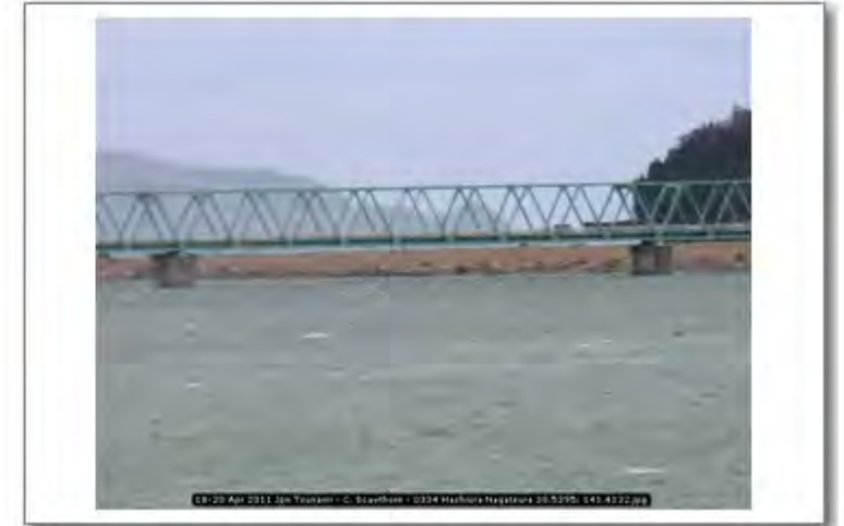
18-20 Apr 2011 Jpn Tsunami - C. Scawthorn - 0334 Hashiura Nagatsura 38.5395; 141.4132
