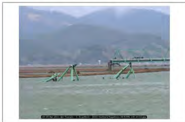
18-20 Apr 2011 Jpn Tsunami - C. Scawthorn - 0832 Hashiura Nagatsura 38.5395; 141.4132
