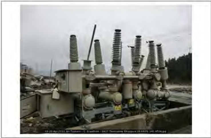
18-20 Apr 2011 Jpn Tsunami - C. Scawthorn - 0427 Tennoumae Shizugawa 38.6809; 141.4536
