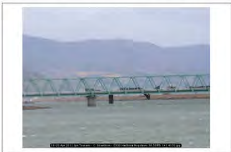
18-20 Apr 2011 Jpn Tsunami - C. Scawthorn - 0330 Hashiura Nagatsura 38.5395; 141.4132
