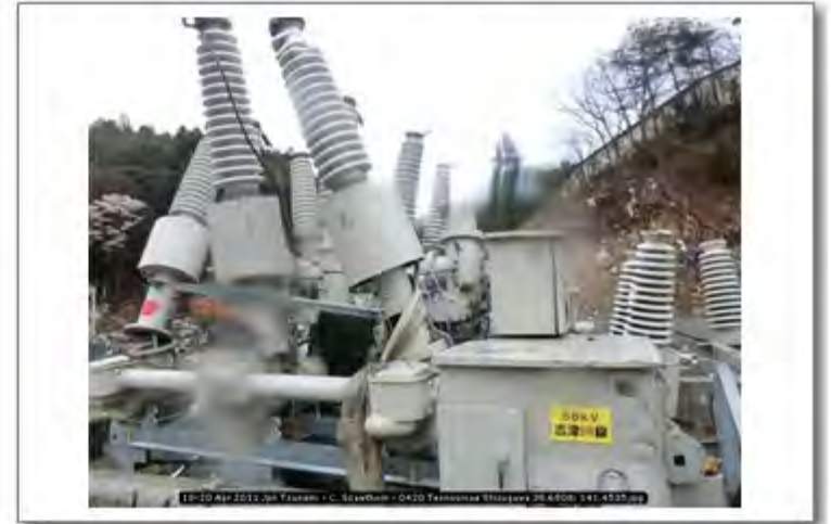
18-20 Apr 2011 Jpn Tsunami - C. Scawthorn - 0420 Tennoumae Shizugawa 38.6808; 141.4535
