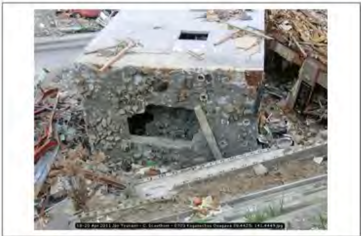
18-20 Apr 2011 Jpn Tsunami - C. Scawthorn - 0703 Koganechou Onagawa 38.4425; 141.4449
