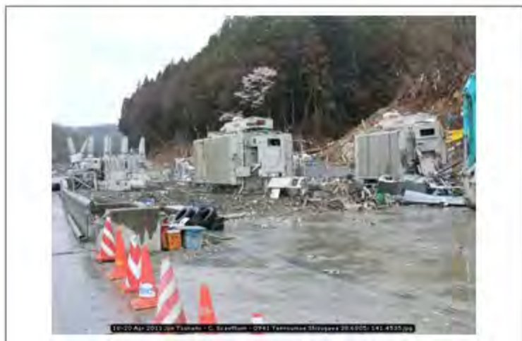
18-20 Apr 2011 Jpn Tsunami - C. Scawthorn - 0941 Tennoumae Shizugawa 38.6805; 141.4535
