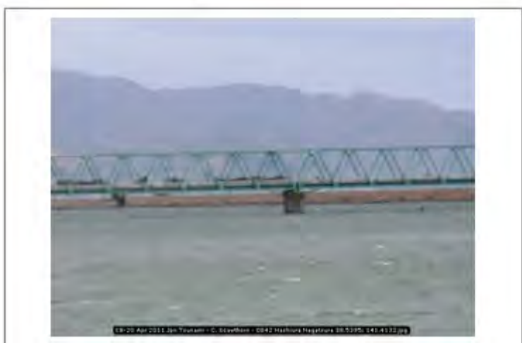
18-20 Apr 2011 Jpn Tsunami - C. Scawthorn - 0842 Hashiura Nagatsura 38.5395; 141.4132
