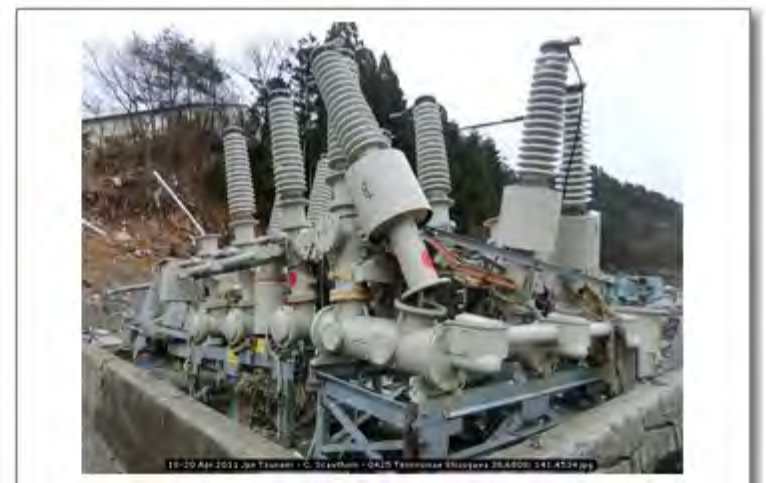
18-20 Apr 2011 Jpn Tsunami - C. Scawthorn - 0425 Tennoumae Shizugawa 38.6808; 141.4534
