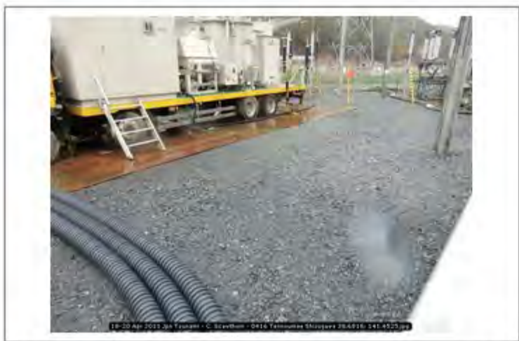
18-20 Apr 2011 Jpn Tsunami - C. Scawthorn - 0416 Tennoumae Shizugawa 38.6818; 141.4525
