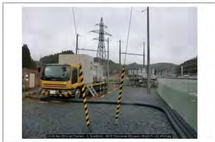
18-20 Apr 2011 Jpn Tsunami - C. Scawthorn - 0415 Tennoumae Shizugawa 38.6817; 141.4524
