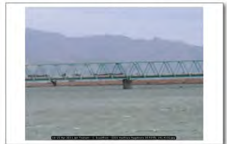
18-20 Apr 2011 Jpn Tsunami - C. Scawthorn - 0331 Hashiura Nagatsura 38.5395; 141.4132
