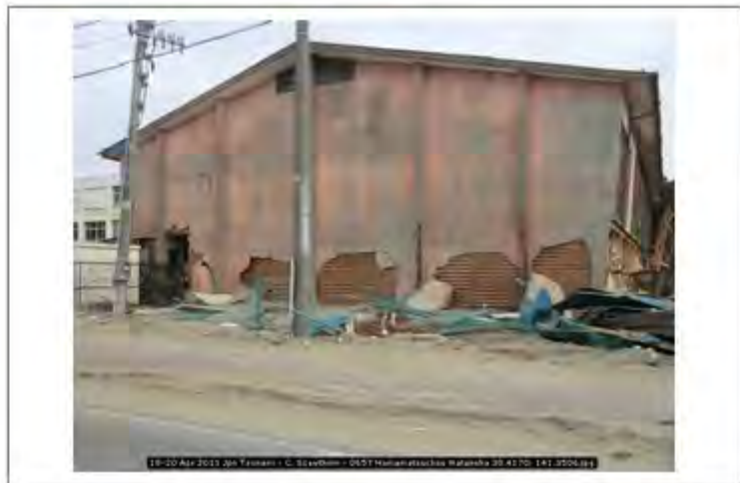
18-20 Apr 2011 Jpn Tsunami - C. Scawthorn - 0657 Hamamatsuchou Watanoha 38.4170; 141.3506
