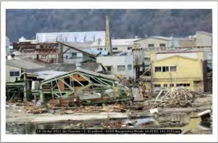
18-20 Apr 2011 Jpn Tsunami - C. Scawthorn - 0109 Myoujinchou Minato 38.4152; 141.3151
