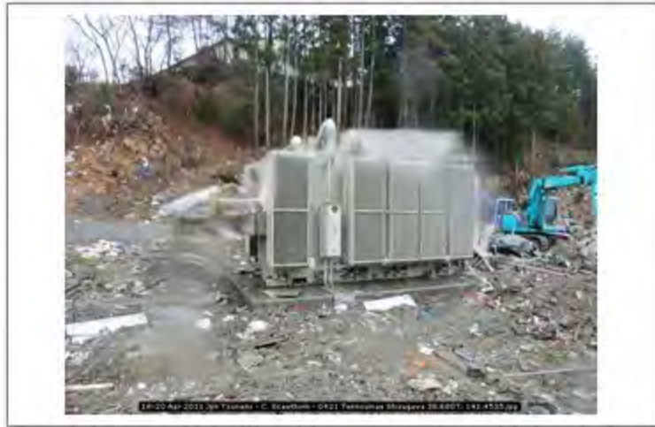
18-20 Apr 2011 Jpn Tsunami - C. Scawthorn - 0421 Tennoumae Shizugawa 38.6807; 141.4535
