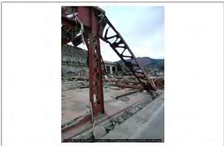
18-20 Apr 2011 Jpn Tsunami - C. Scawthorn - 0733 Koganechou Onagawa 38.4428; 141.4461
