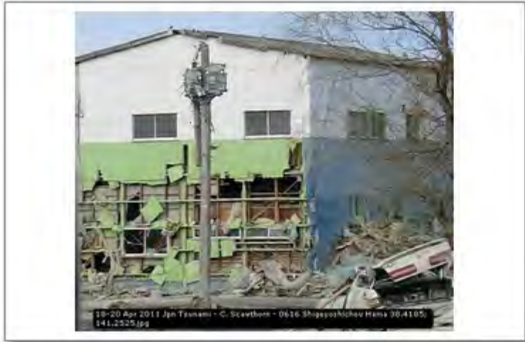
18-20 Apr 2011 Jpn Tsunami - C. Scawthorn - 0616 Shigeyoshichou Hama 38.4185; 141.2525
