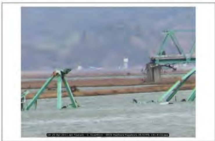
18-20 Apr 2011 Jpn Tsunami - C. Scawthorn - 0833 Hashiura Nagatsura 38.5395; 141.4132
