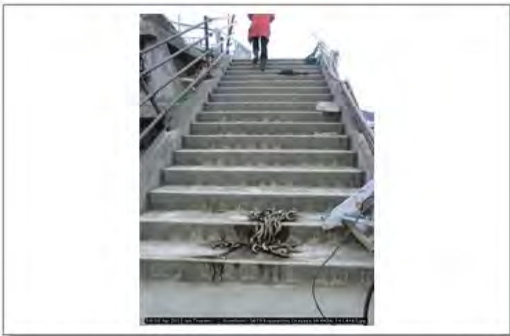
18-20 Apr 2011 Jpn Tsunami - C. Scawthorn - 0679 Koganechou Onagawa 38.4434; 141.4463
