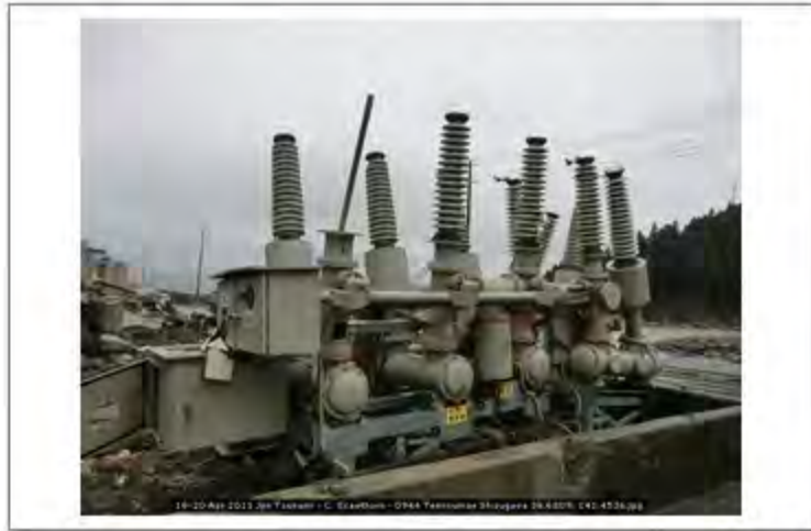
18-20 Apr 2011 Jpn Tsunami - C. Scawthorn - 0944 Tennoumae Shizugawa 38.6809; 141.4536
