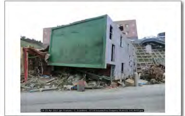
18-20 Apr 2011 Jpn Tsunami - C. Scawthorn - 0716 Koganechou Onagawa 38.4422; 141.4450
