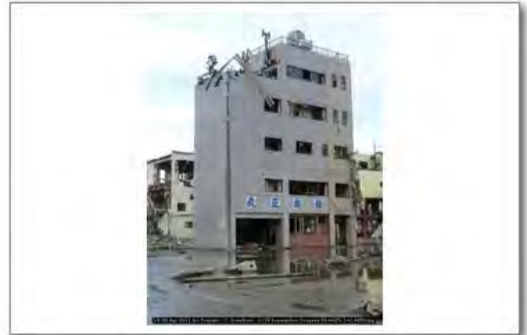
18-20 Apr 2011 Jpn Tsunami - C. Scawthorn - 0174 Koganechou Onagawa 38.4425; 141.4453
