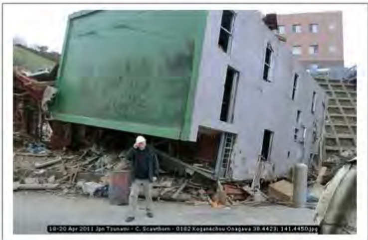
18-20 Apr 2011 Jpn Tsunami - C. Scawthorn - 0182 Koganechou Onagawa 38.4423; 141.4450
