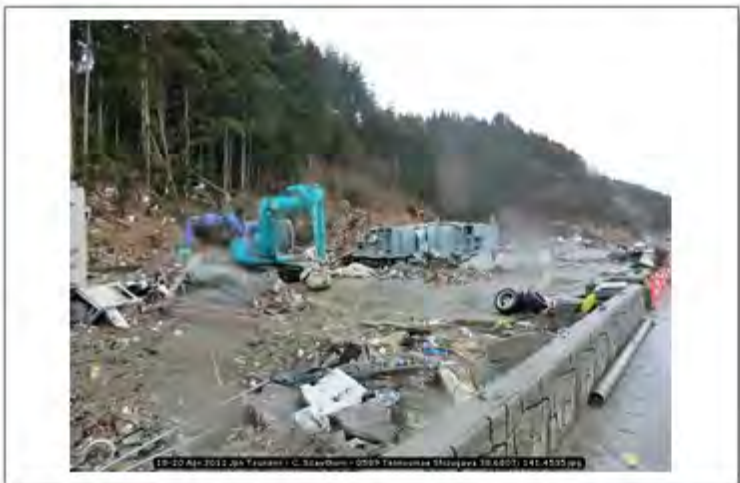
18-20 Apr 2011 Jpn Tsunami - C. Scawthorn - 0589 Tennoumae Shizugawa 38.6807; 141.4535
