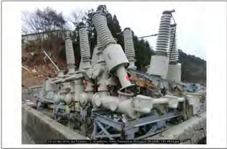
18-20 Apr 2011 Jpn Tsunami - C. Scawthorn - 0942 Tennoumae Shizugawa 38.6808; 141.4534
